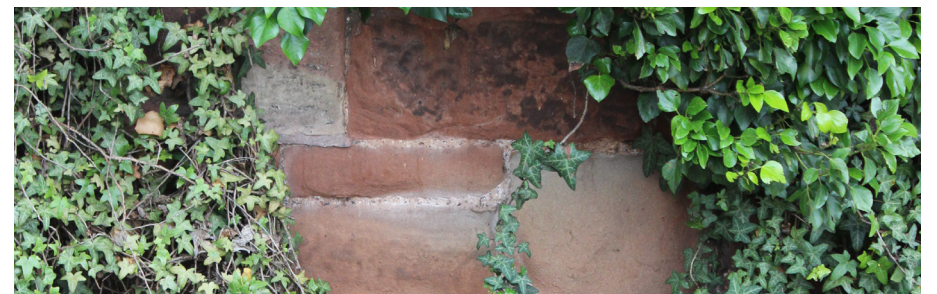
Figure 23 The contrast between the red sandstone of the bank and the greenery which lines Wightwick Bank is visually attractive and an important feature of the Conservation Area.
